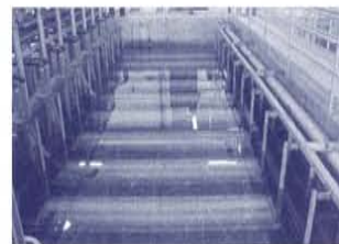
Membrane cassettes in MBR tank.
